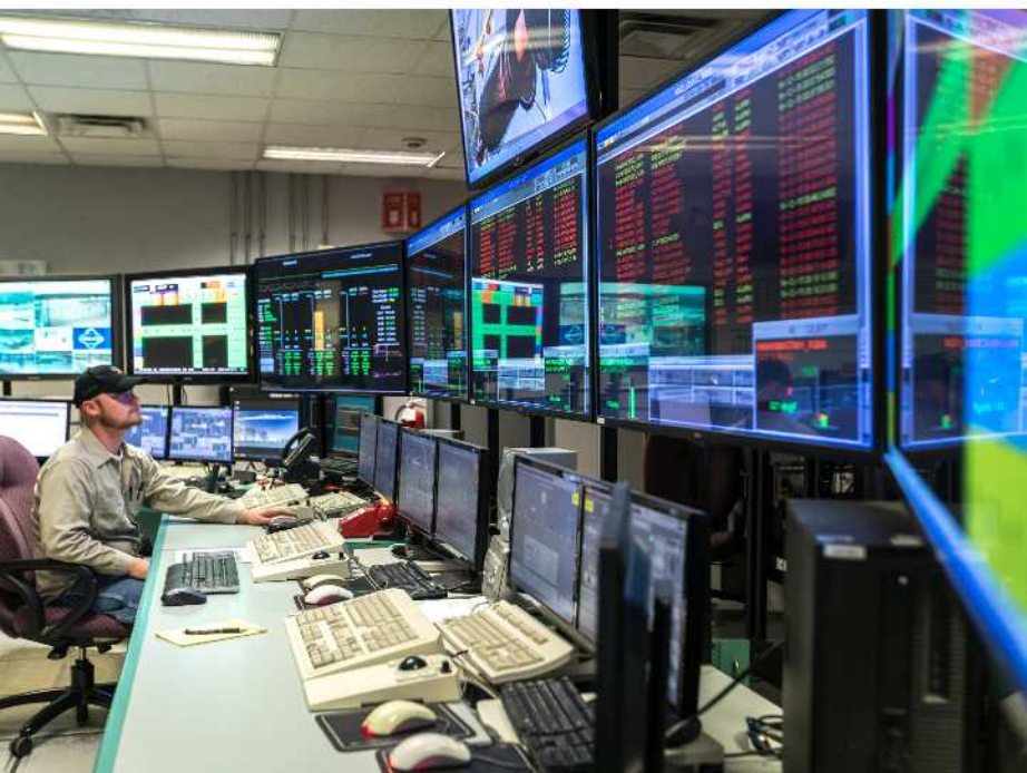
A control room operator monitors the electricity generating systems at one of Vistra's 50 power plants, which produce enough power for 20 million homes.
