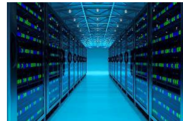
Stationary backup and prime power: Data centers as early adopters
